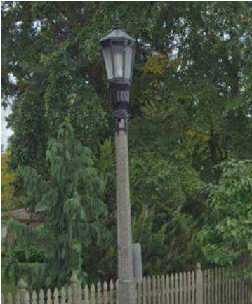
Current post-top fixture (13 ft. high):
