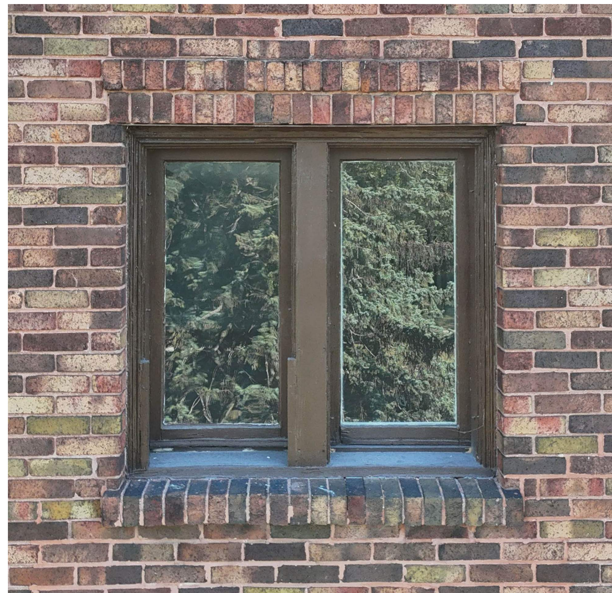
NON-HISTORIC REPLACEMENT WINDOWS
