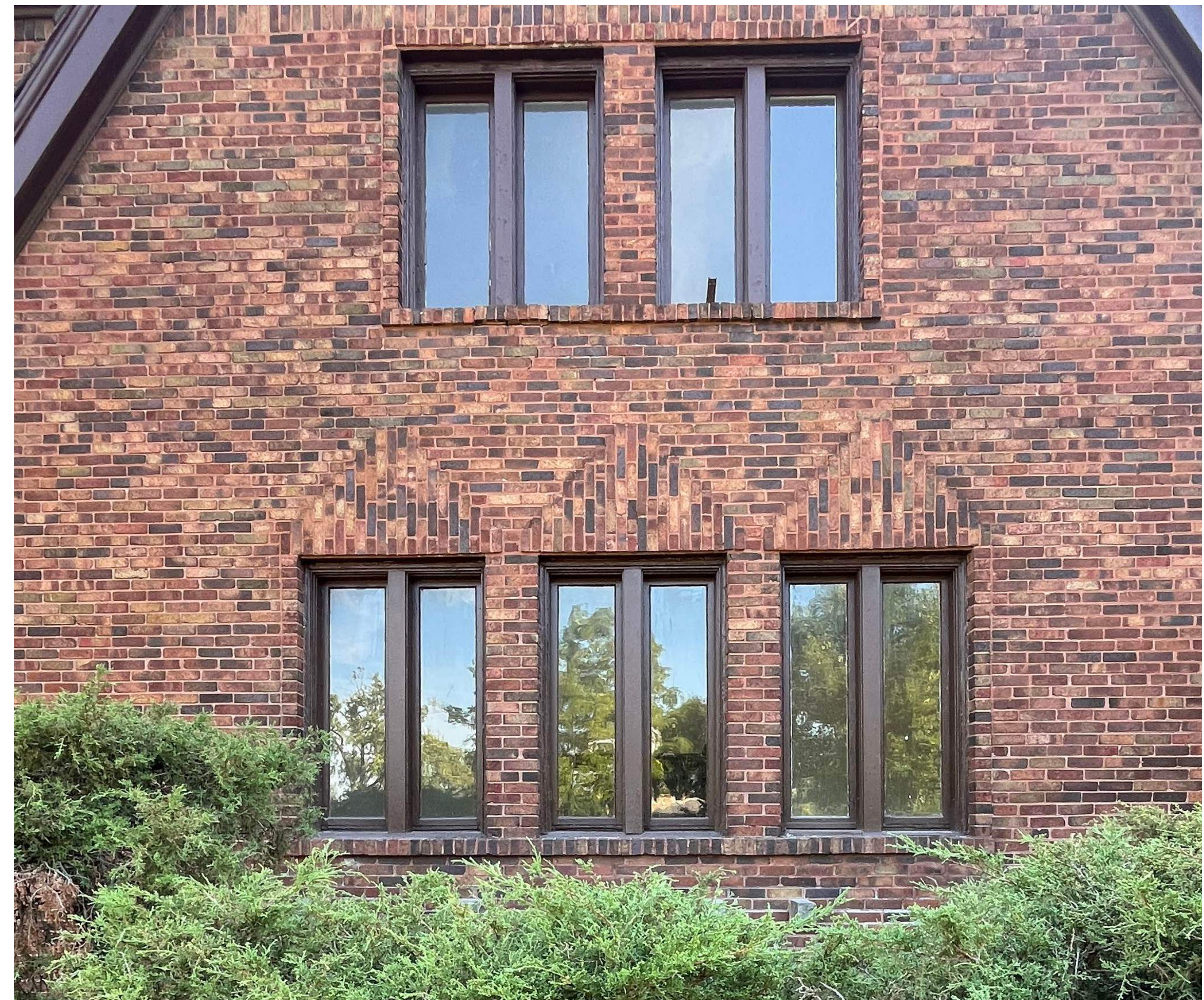
NON-HISTORIC REPLACEMENT WINDOWS
