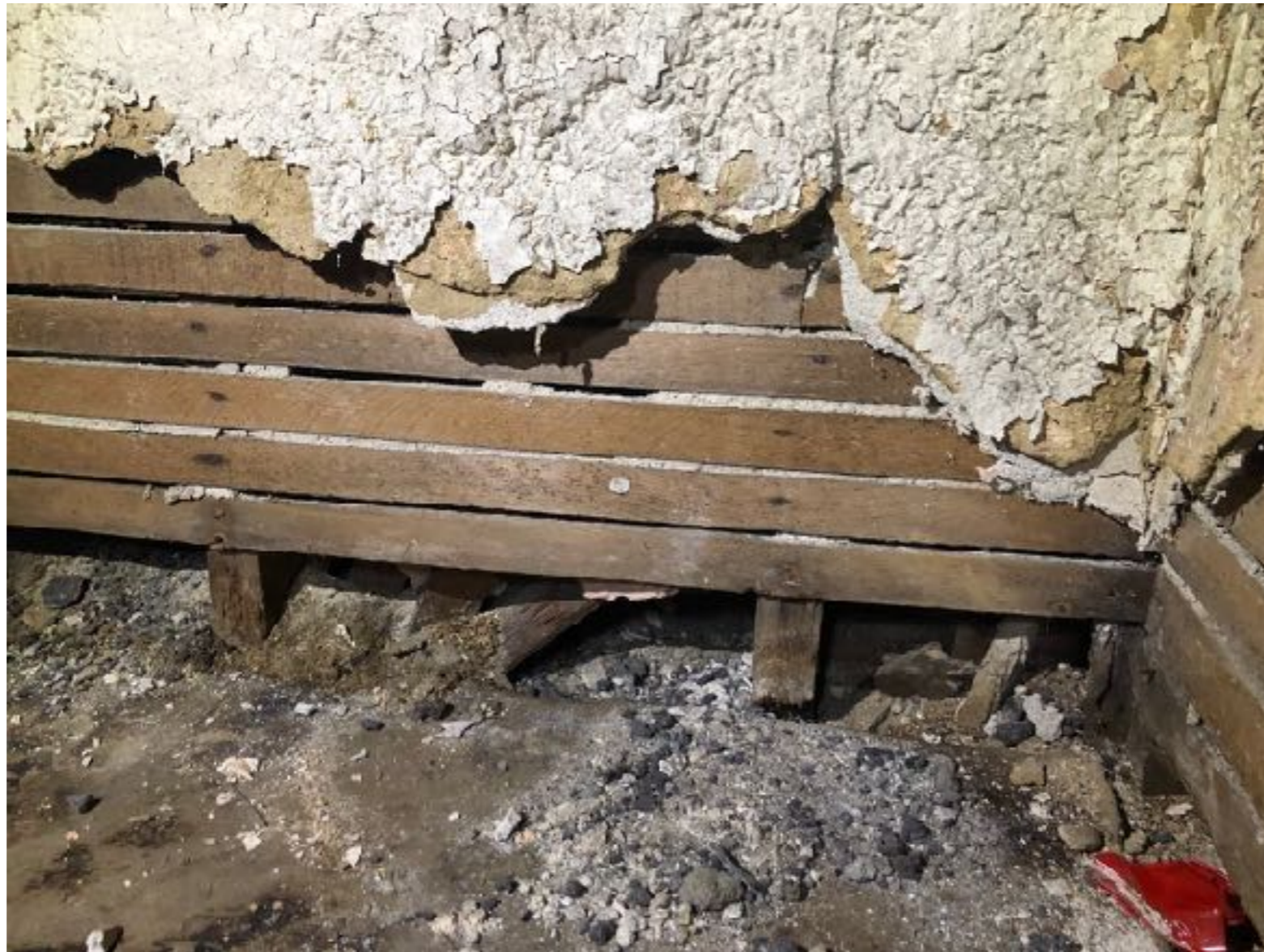
SLAB MISSING WOOD ROT AT BEARING WALL
