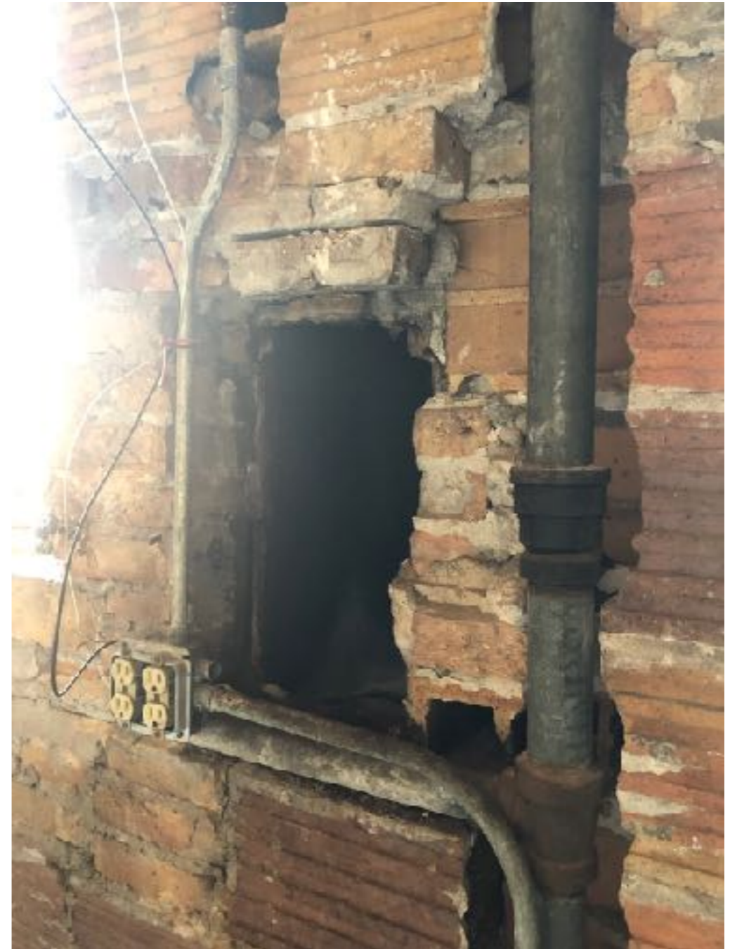
EXTERIOR BEARING WALL DISREPAIR
