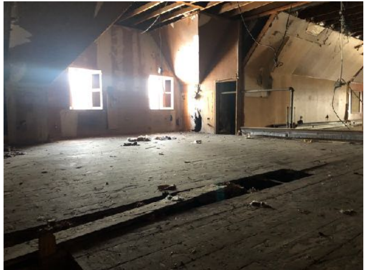
FLOOR SAGGING AND DISPLACEMENT
