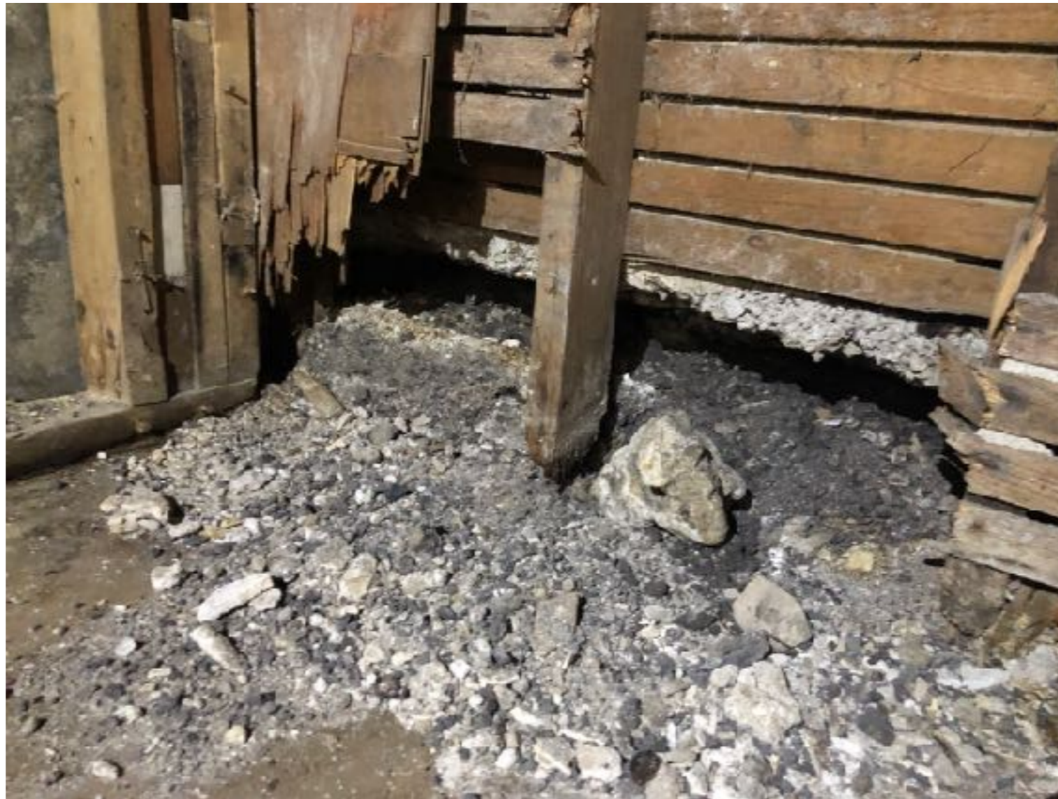
SLAB MISSING WOOD ROT AT BEARING WALL
