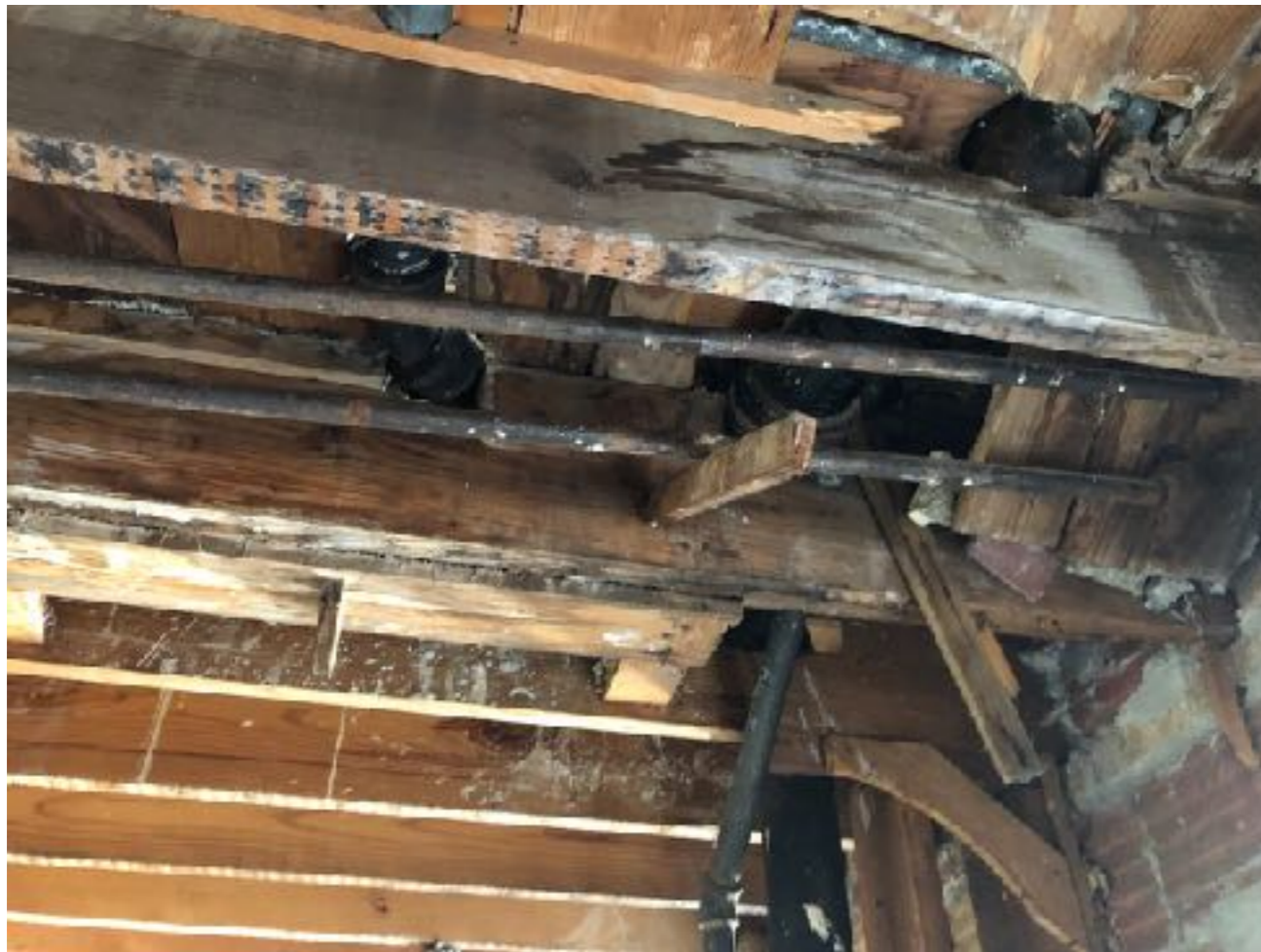
WOOD ROT STRUCTURAL DISREPAIR
