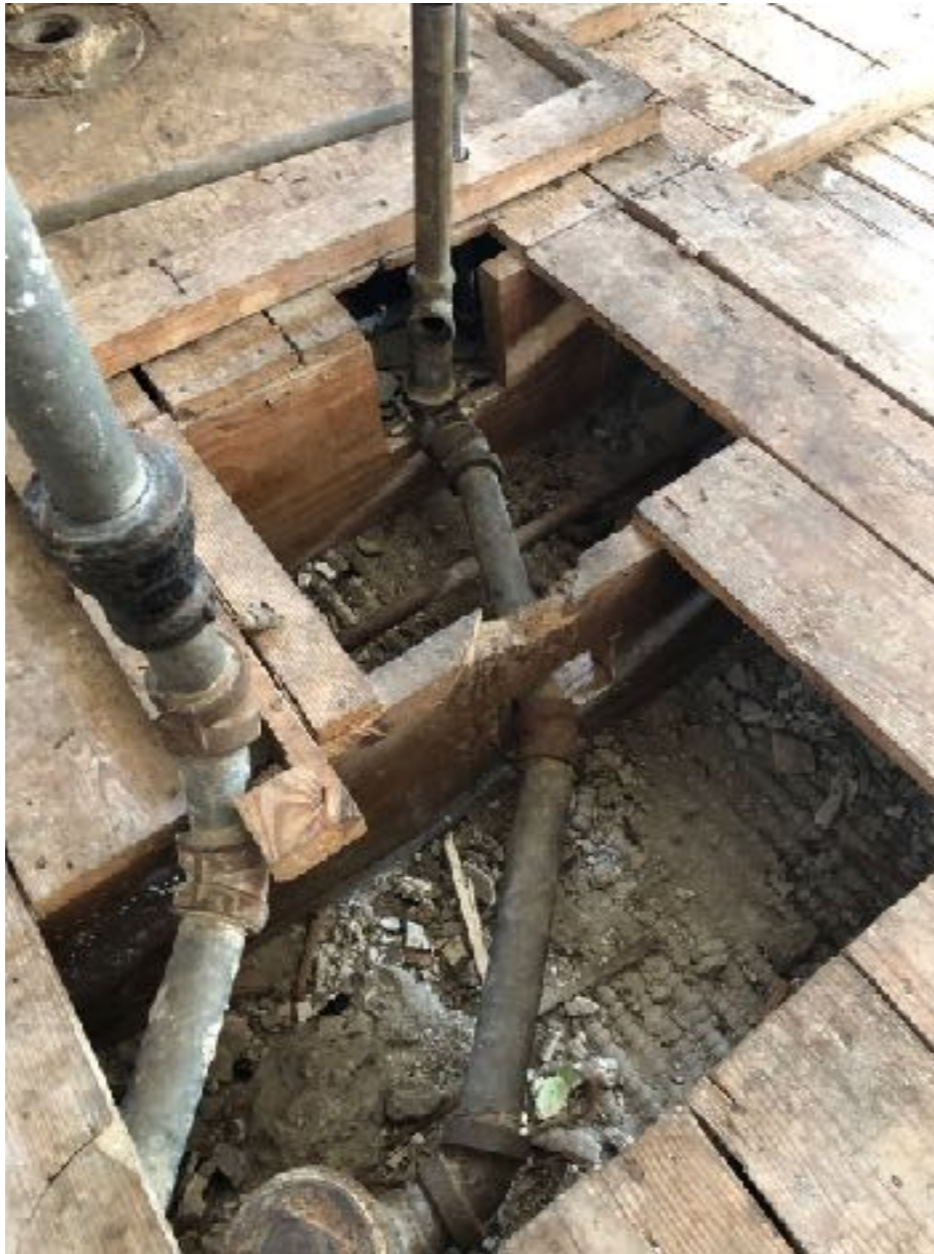
STRUCTURAL DAMAGE TO FLOOR JOISTS
