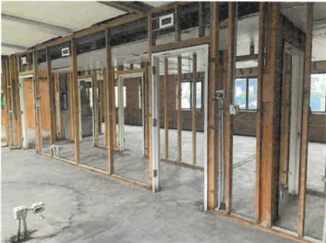
7620 W Madison River Forest, II Drywall wall board and joint compound removed
