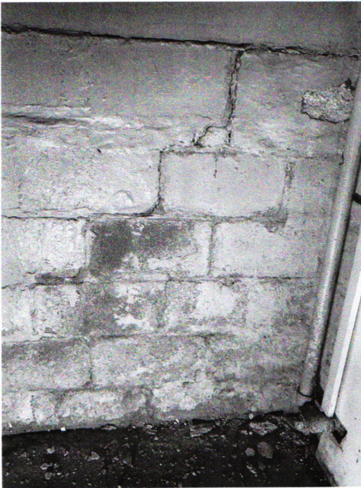
Photograph #2 - Foundation wall crack, southeast corner
