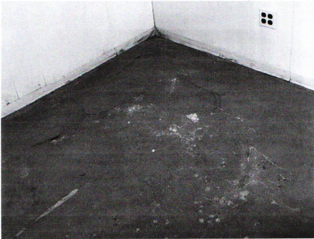
Photograph #10 - heaved floor slab in northwest corner of basement
