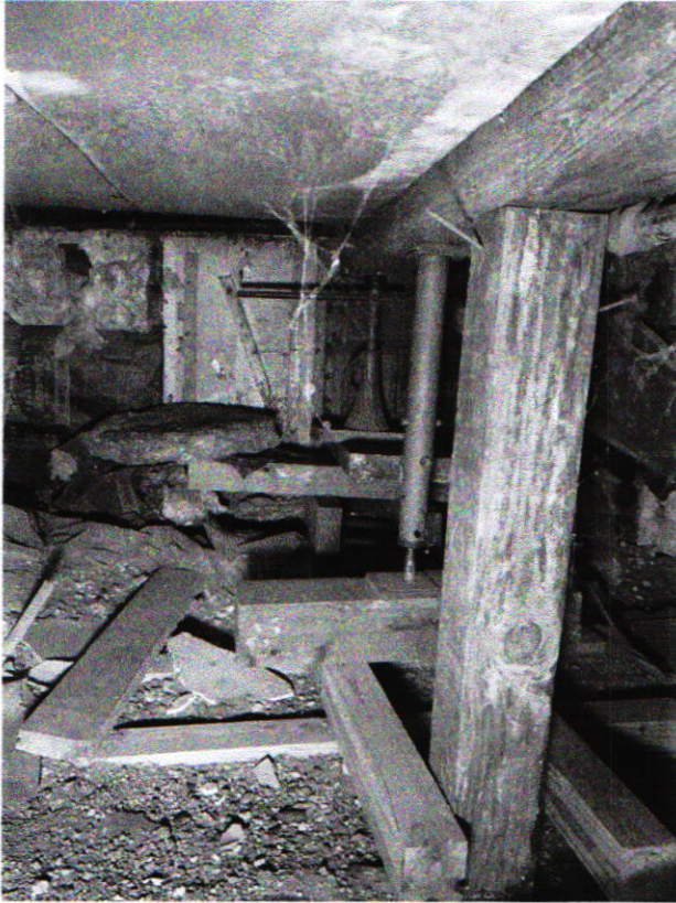
Photograph #7 - shoring & posts below southeast corner area
