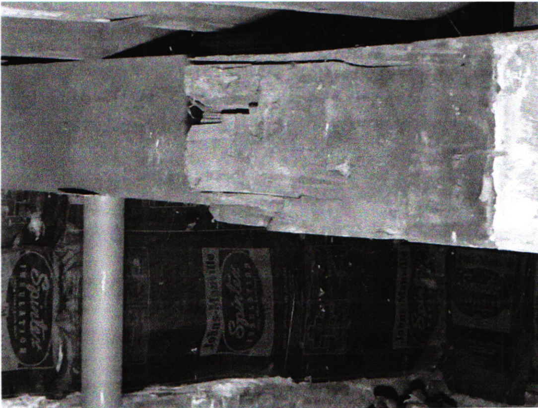
Photograph #6 - unsupported beam end under sun porch
