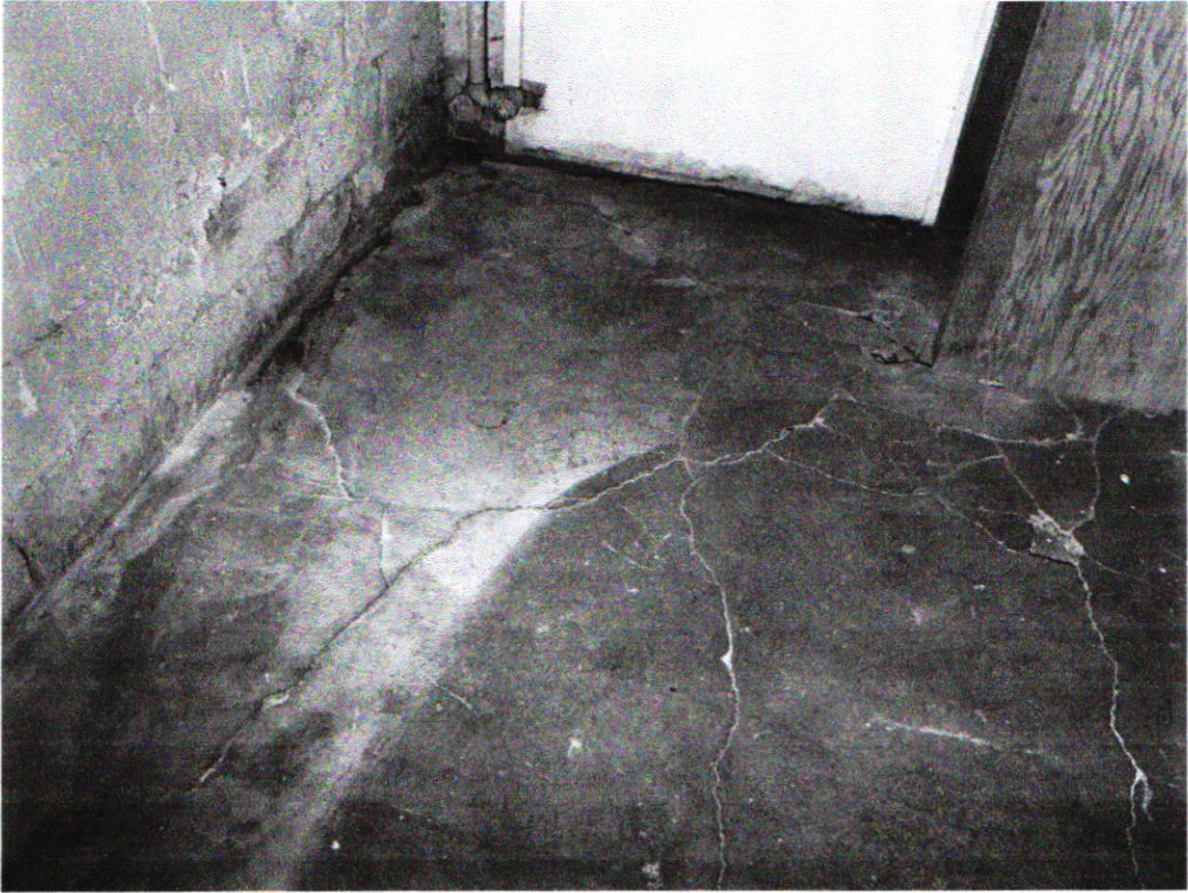
Photograph #11 - heaved floor slab in southeast corner of basement
